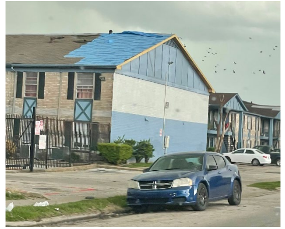
Tarps cover the damaged roof of an apartment complex in Houston.
