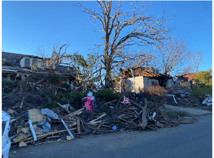
Layers of debris in Mayfield, Kentucky, require multiple phases of removal to ensure safe access to roads and power lines.
